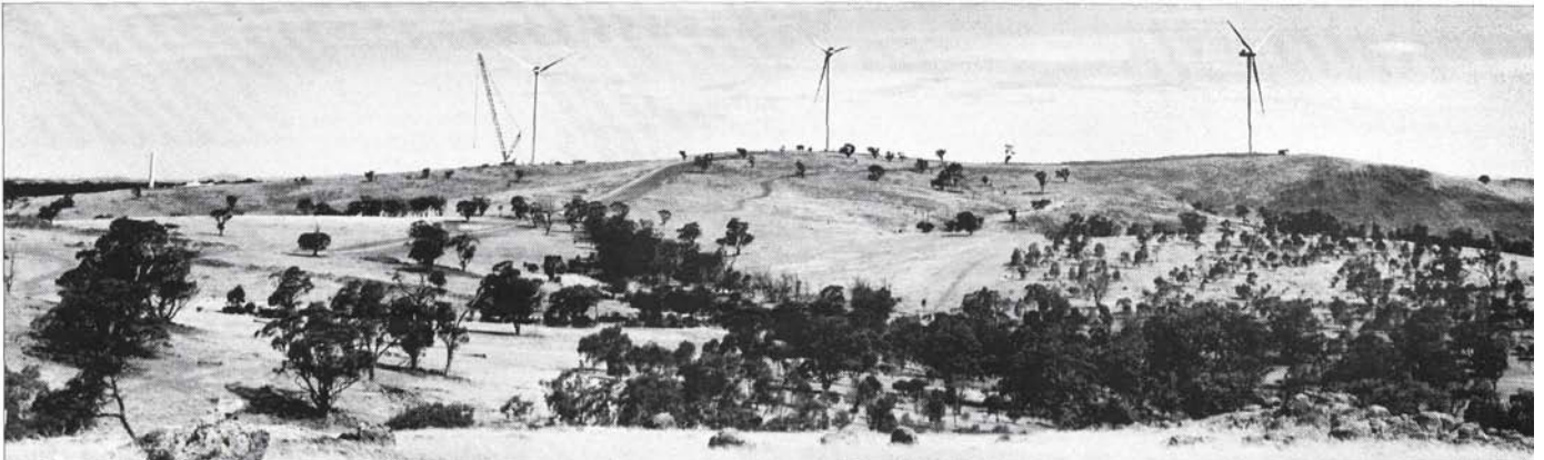
• The changing landscape – pictured dotted across a section of the wind farm site are from the left Towers 1 (extreme left partially erected), 2, 3 and 4.
